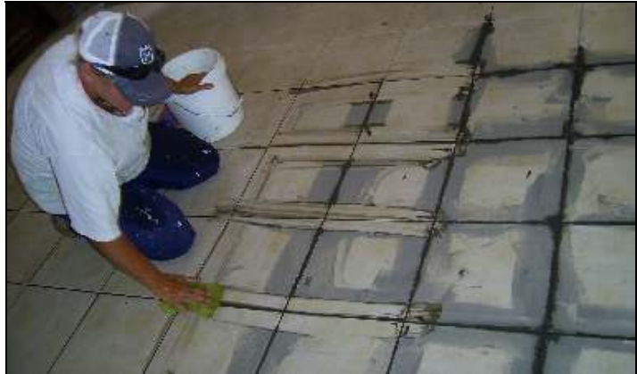
Karen is grouting floor tiles in the new entrance of the Café
